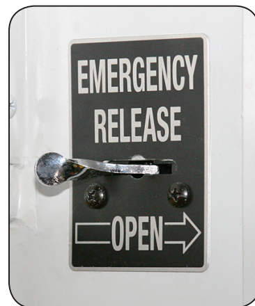
Air Door Emergency Release
